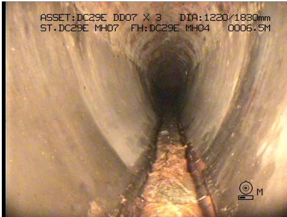
Figure 4: Photograph Taken Inside the Tank Stream Drainage Structure Between Access Chambers AC7 and AC4
