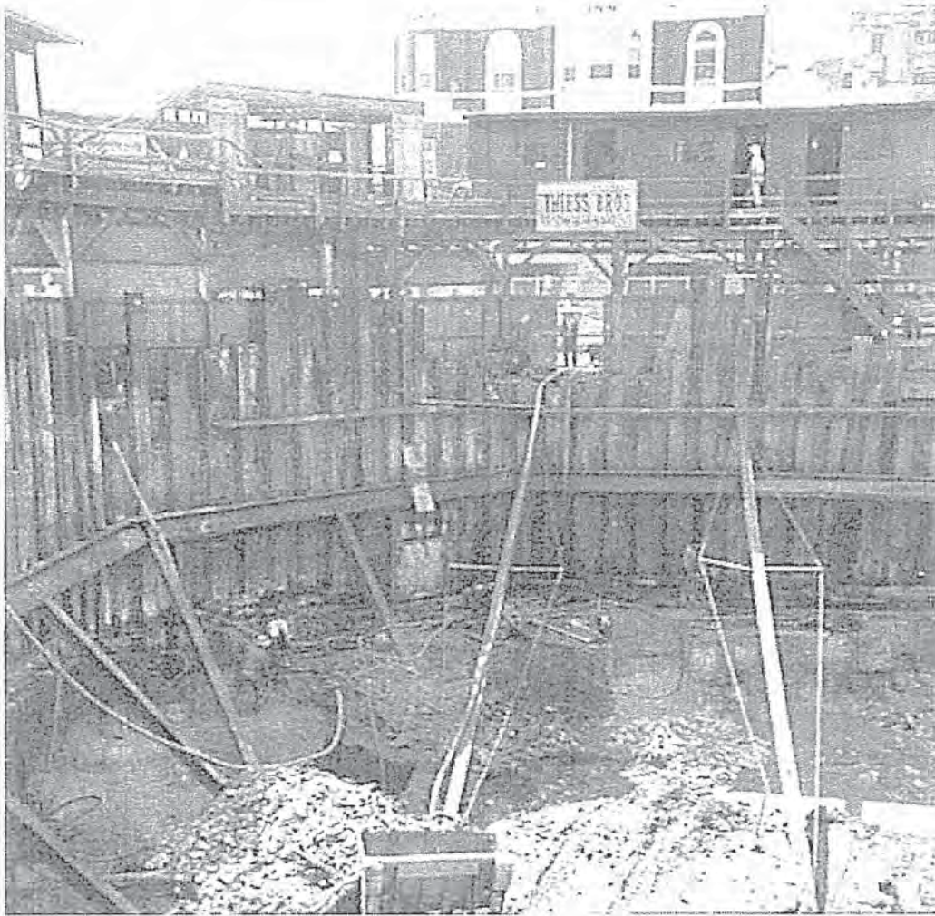
Figure 2.15 1965 image showing the excavation and shoring for the below ground levels of the Gold Fields House development. This view is looking east to Pitt Street, note the bystander on street level (beneath the Theiss sign). The tank stream is in Pitt Street behind the shoring. (Source: City of Sydney Council Archive)
